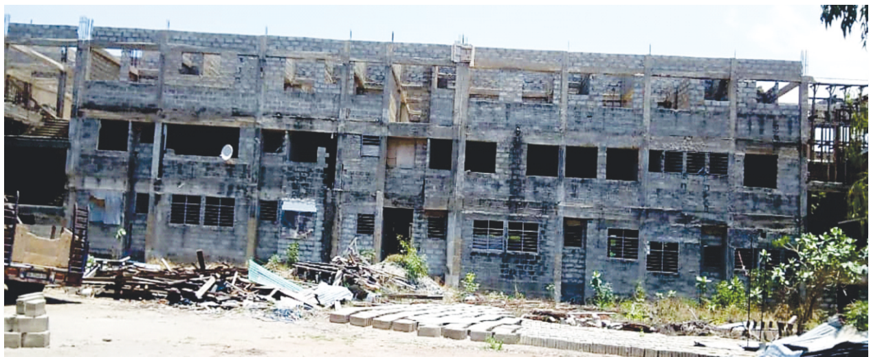
Abandoned maternity block at Tema General Hospital. Even though the project started in April 2010, only 55% of work has been done within 8 years as we are in 2019
