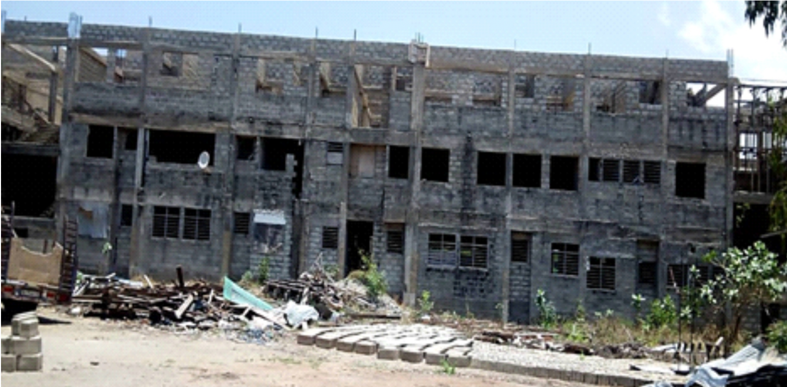
Abandoned Maternity Block at Tema General Hospital
