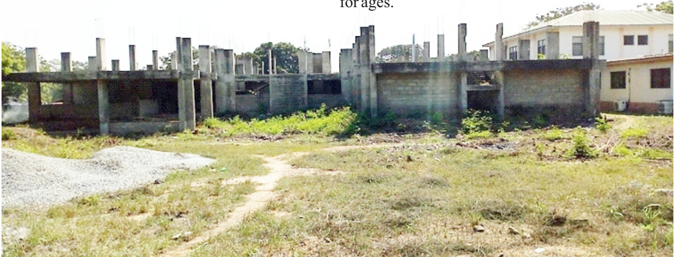
Stalled Regional Health Directorate Project located at Adabraka. The project started in October 2004 and was to be completed in December, 2006 but only 38% of work had been done till date
